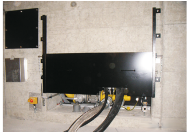
Connection Point for Gas and Power
