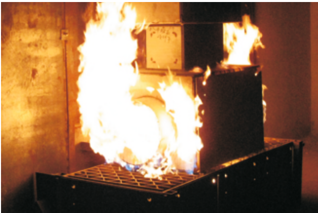
Motor Generator Fire
