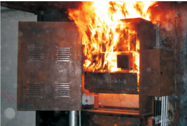
Electrical Panel Fire
