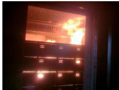
Motor Control Center Fire
