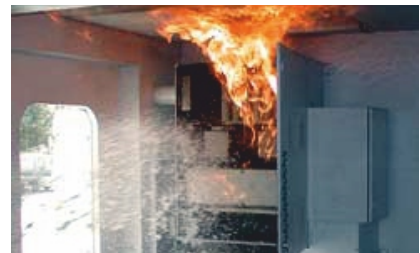
Electrical Panel Fire
