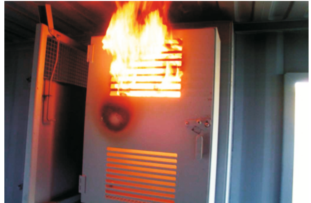
Electrical Panel Fire
