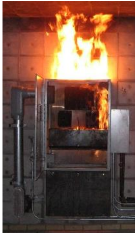
Electrical Panel Fire
