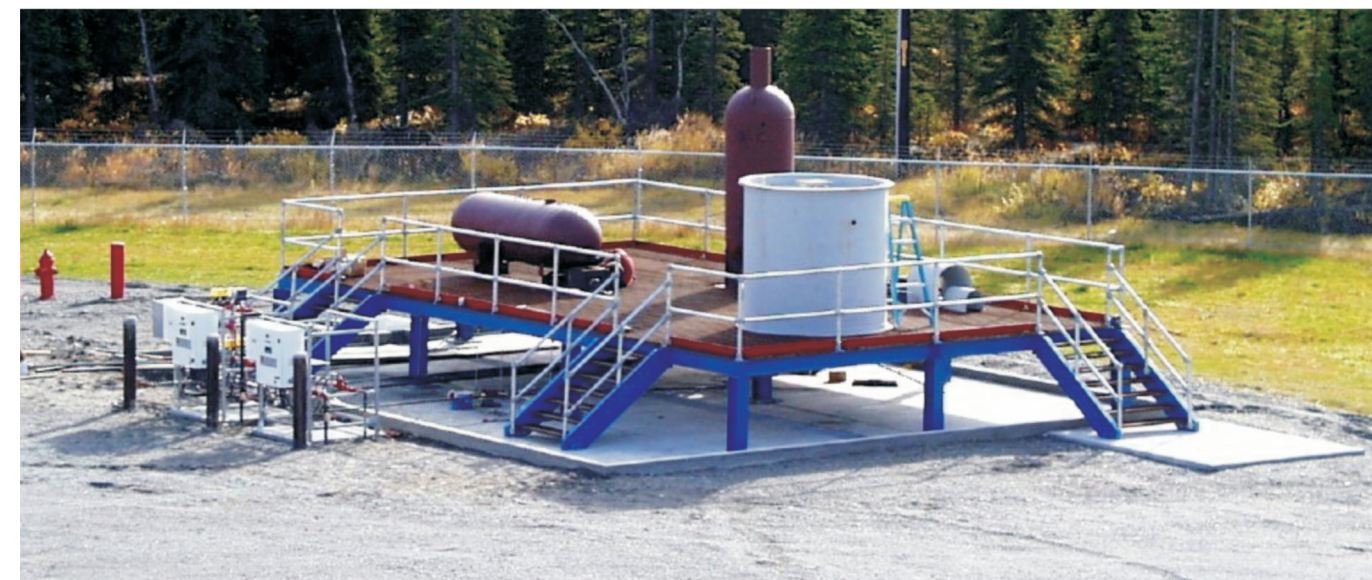
raised industrial platform
