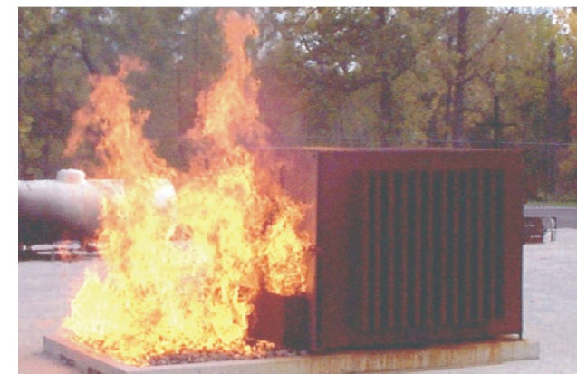
leaking transformer fire
