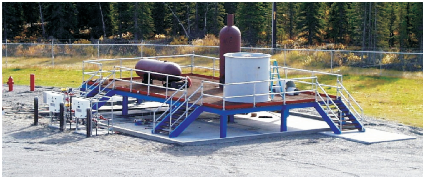
raised industrial platform
